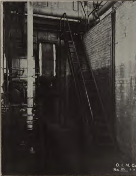
No. 8—Sec. 16 Boiler House, Ishpeming, Mich.
